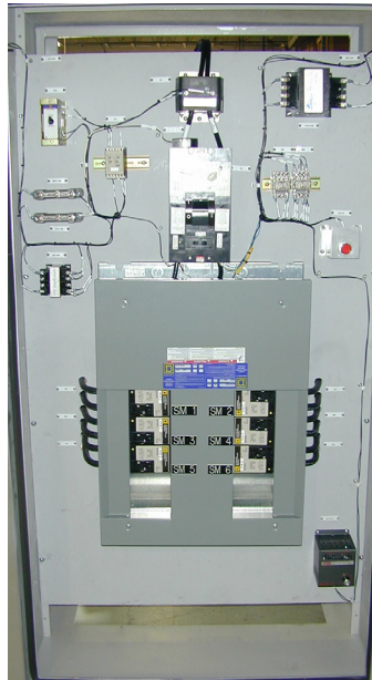
MNCRR 480VAC, 6 Circuit Controller
